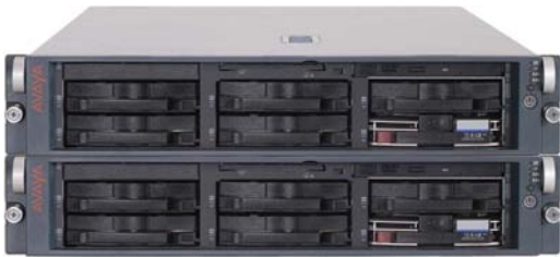
Figure 1: Avaya S8710 Media Servers
